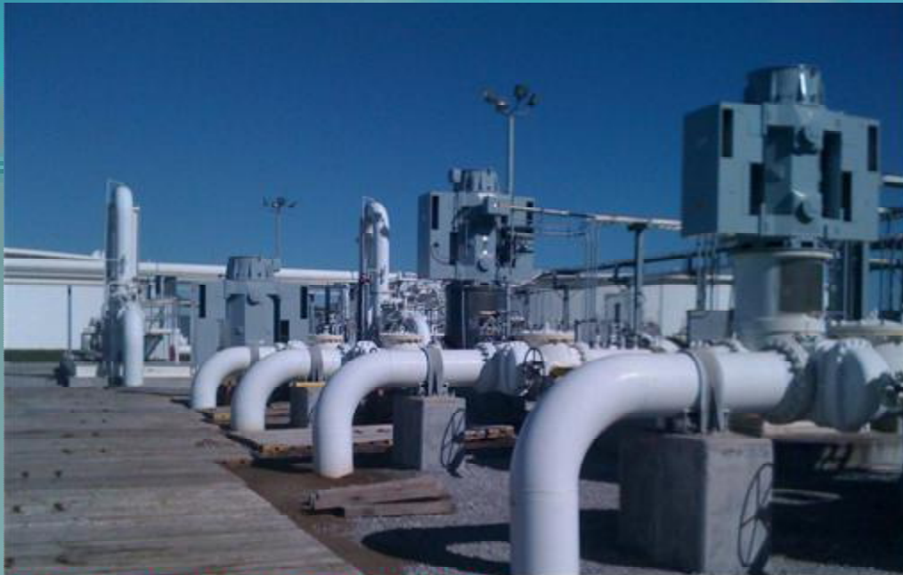
Pipeline Booster Station (Cloveley, Louisiana)
